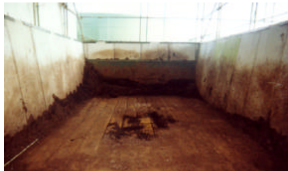
Fig. 6. In-vessel bunker with aeration system on the floor.
