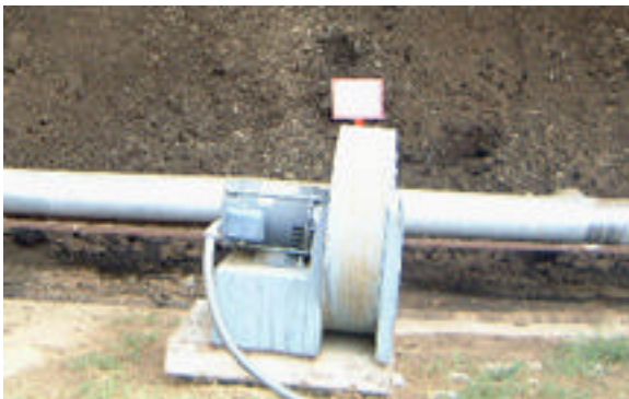
Fig. 3. Fan used to aerate composting pile.
